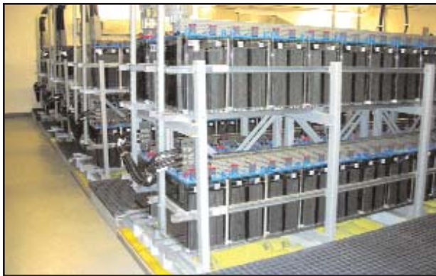
Figure 1. Typical large flooded lead acid battery system
