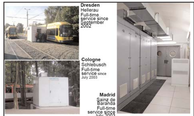
Figure 5. SITRAS SES Installation Examples
