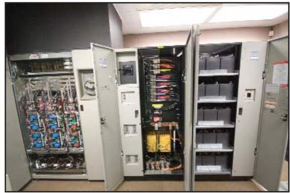
Figure 2. It is extremely important to make sure batteries are operating properly and within manufacturers' specifications. In fact, your battery warranty may even be voided if proper maintenance is not provided.
