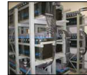
Batteries Play Role in Green Data Center, page 12
