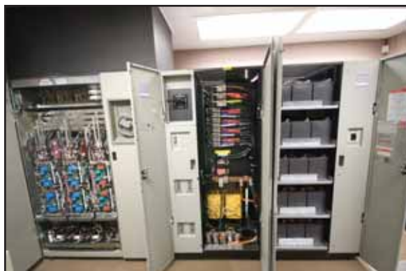
Figure 2. It is extremely important to make sure batteries are operating properly and within manufacturers' specifications. In fact, your battery warranty may even be voided if proper maintenance is not provided.
